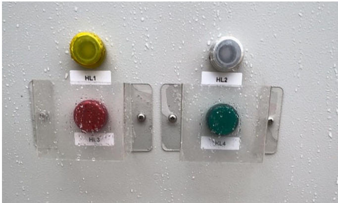
1# AC combiner cabinet
